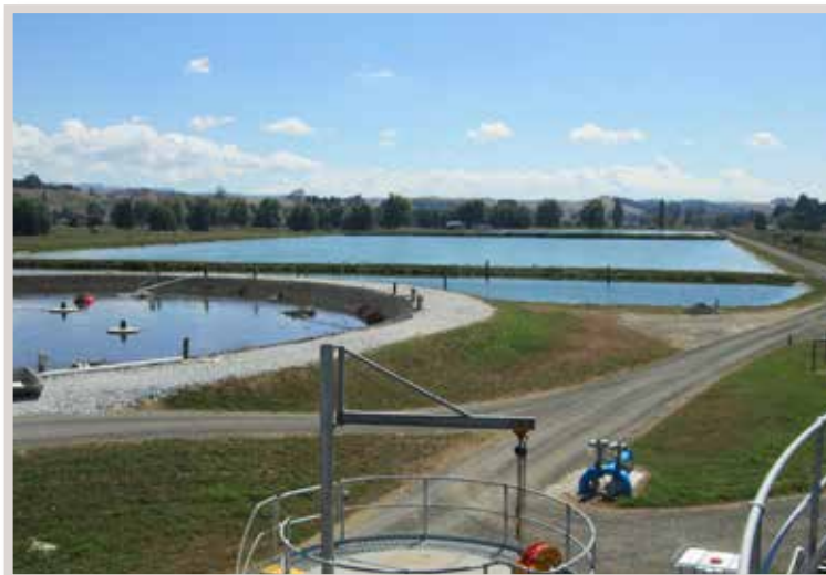
OVERVIEW - TE KUITI WASTE WATER TREATMENT PLANT
