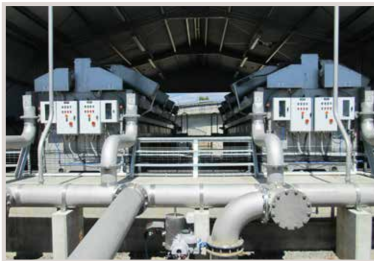
FILTRATION SYSTEM - TE KUITI WASTEWATER TREATMENT PLANT
